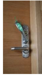
Pic. 5.5.1 emergency lock
