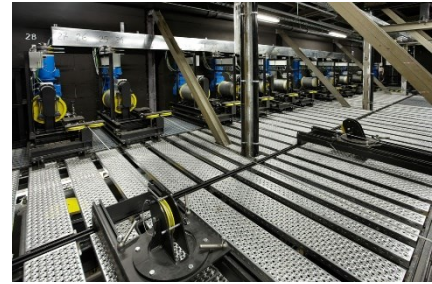
Pic. 10.3.12 Point hoists
